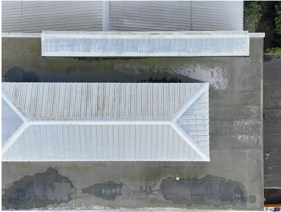
Paired visual frame — organic growth and wet staining along the channel; outlet visible lower right within a stained zone.
