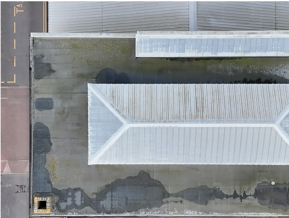
Paired visual frame — dark moisture staining matching the thermal anomaly pattern.
